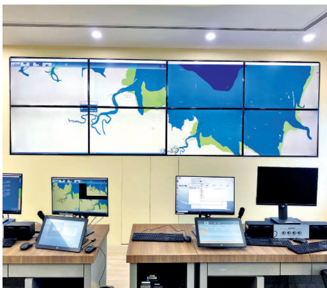
Bilik Kawalan VTMS VTMS Control Room
